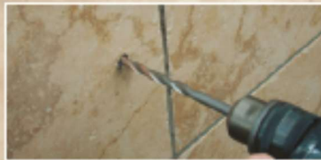
A hole is being produced in the substrate behind the tile with a suitable drill bit for the material being drilled
